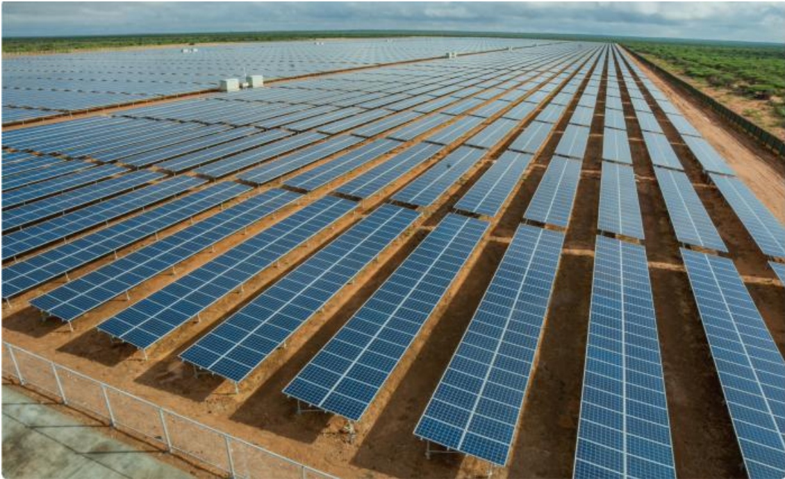
Figure 3.5: Garissa solar power plant (Jan March Newsletter Quater 3, 2021)
