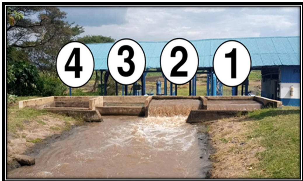
Figure 3.7: Pumping station: Discharge outlets for Pump 1, Pump 2, Pump 3, and Pump 4
