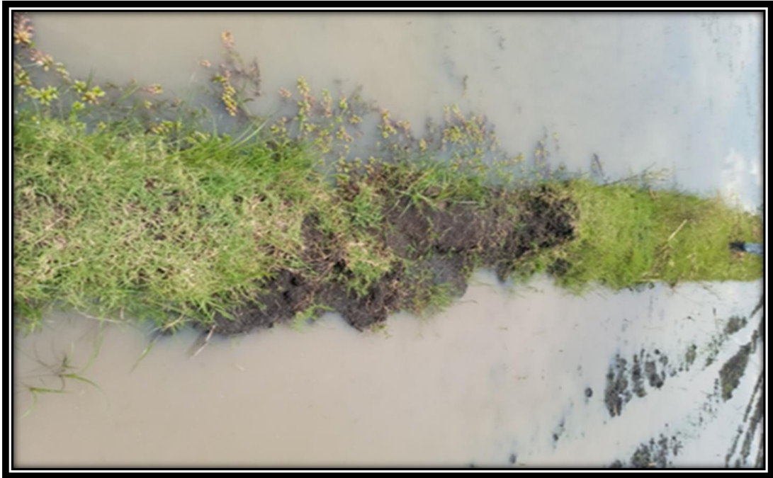
Figure 4.9: Broken basin bunds
