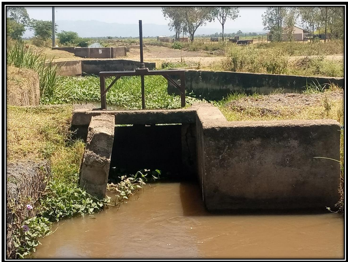
Figure 4.3: Failing water control structure – Division box
