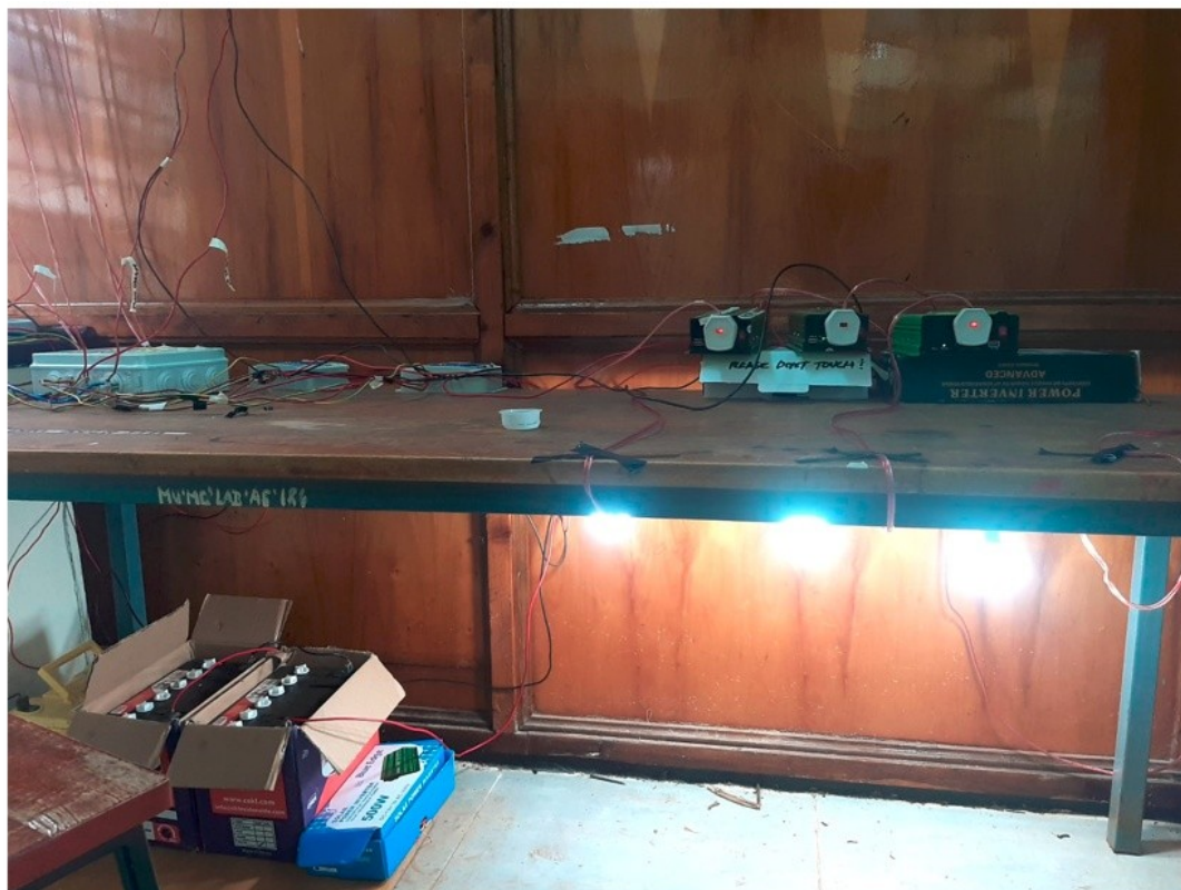
Figure 3.12: Inverter and load (bulbs)
