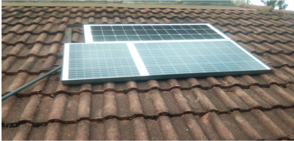
Figure 3.9: PV panels on the clear roof
