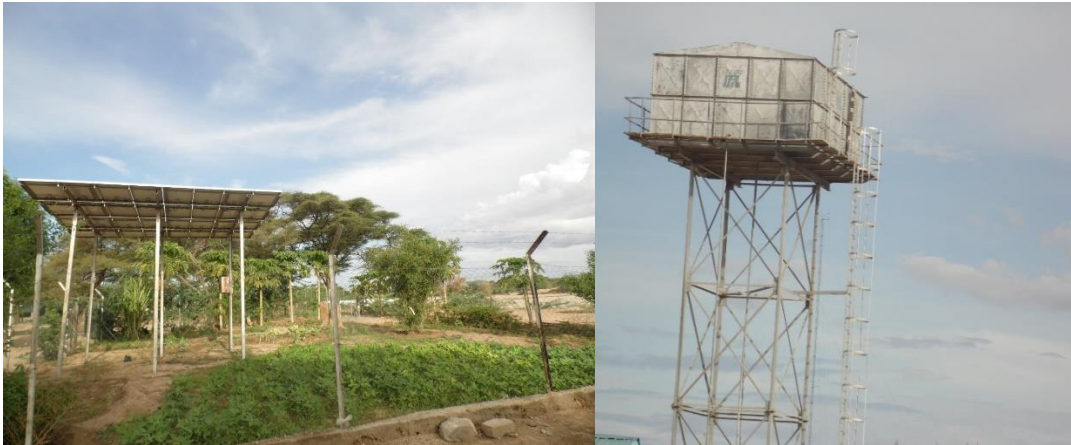
Plate 6: Solar Panels to Pump Water at Kalapata
