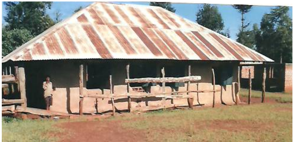
Figure 4.4: A sampled school to illustrate poor ventilation. A classroom with poor ventilation at a primary school in Nandi central district .
