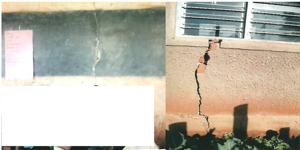
Figure 4.6: Sampled school to illustrate the state of the walls which posed insecurity to the users.
