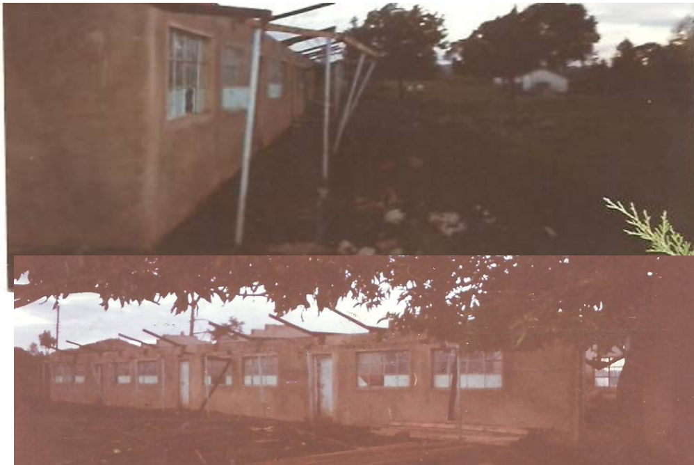
Figure 4.1: A school block destroyed by wind at a primary school in Nandi Central District
