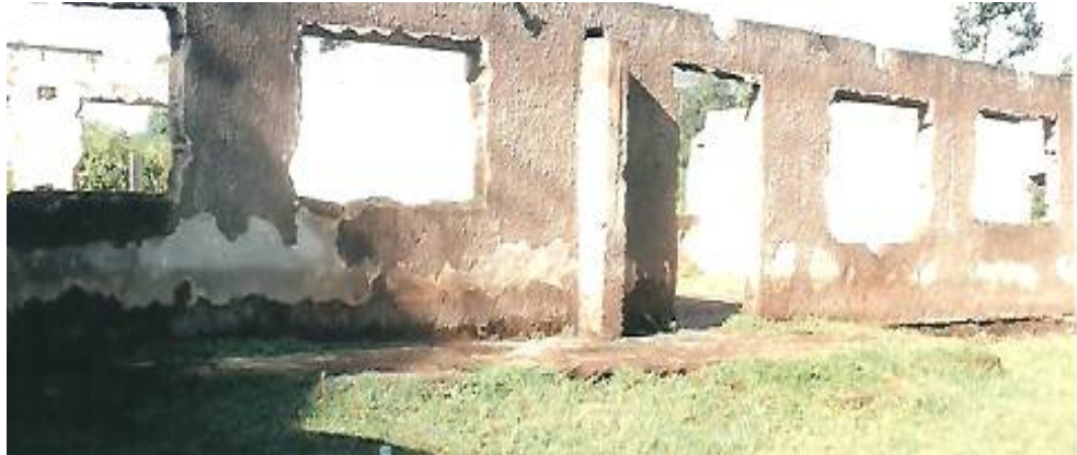
Figure 4:2 Sample school to illustrate a demolished block as a result of cracks
