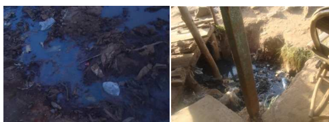
Figure 4.2: the drainage system in West market place
