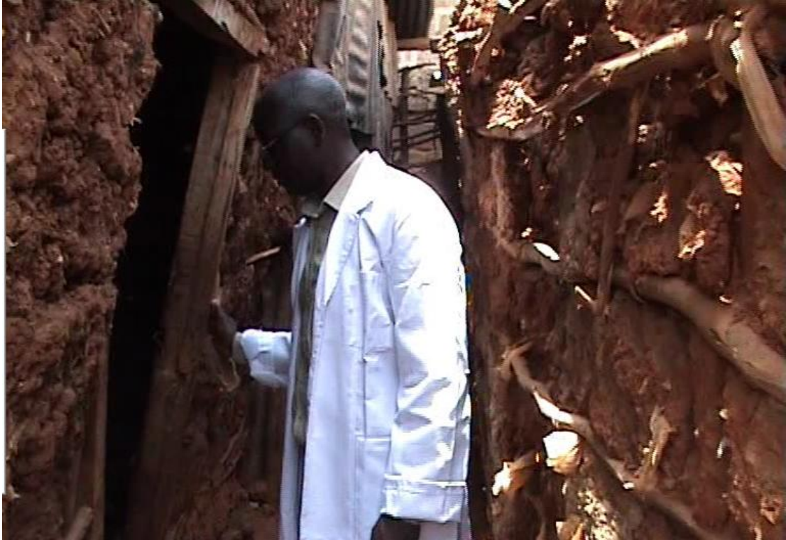
Deplorable Housing state at Kibera slum; mud and wattle this is.
