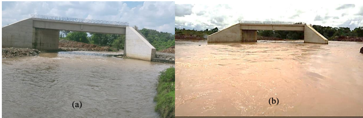
Figure 5: (a) Bridge under construction showing water levels during dry and (b) rainy seasons.
