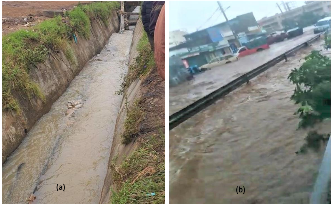
Figure 4: (a) Lined drainage canal before heavy rainfall and (b) after a heavy rainfall causing flooding.
