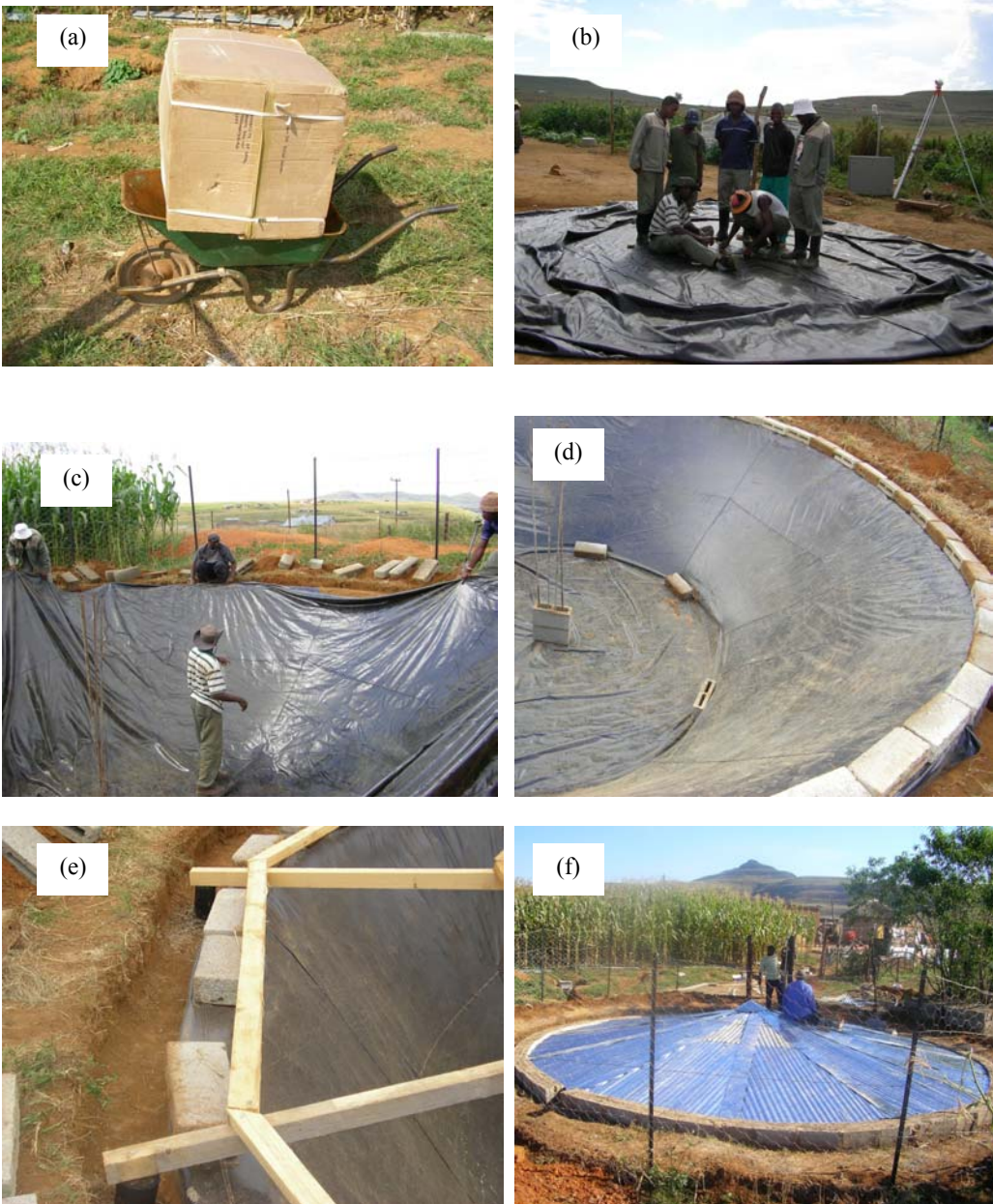
Figure 7.8: Steps of construction of an underground truncated cone RHST – a) plastic liner before being unpacked; b) marking out slots to allow for steel reinforcement in king post; c) and d) laying of liner; e) timber truss; and f) roofing with corrugated iron sheets
