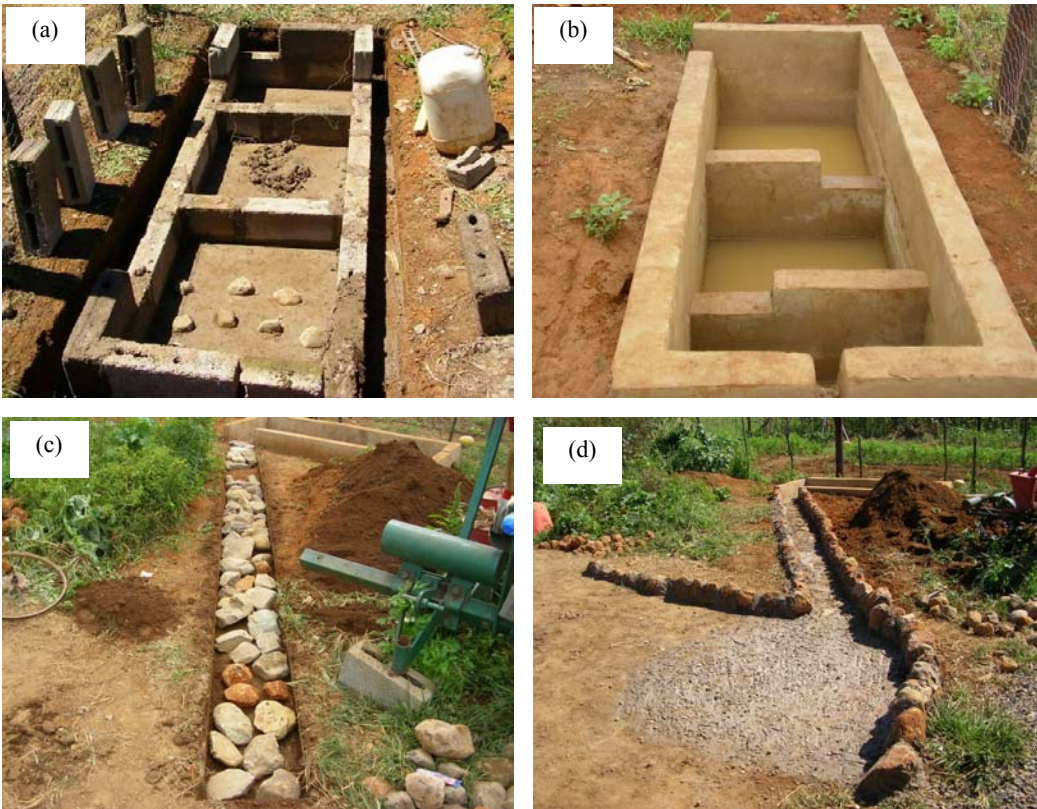
Figure 7.5: Sediment trap and its accessories (a) construction; (b) complete trap; (c) construction of runoff conveyance channel; and (d) runoff concentration area
