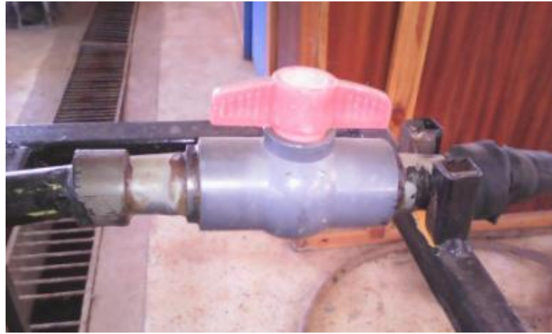
Figure 4.3 (a): Flow control valve
