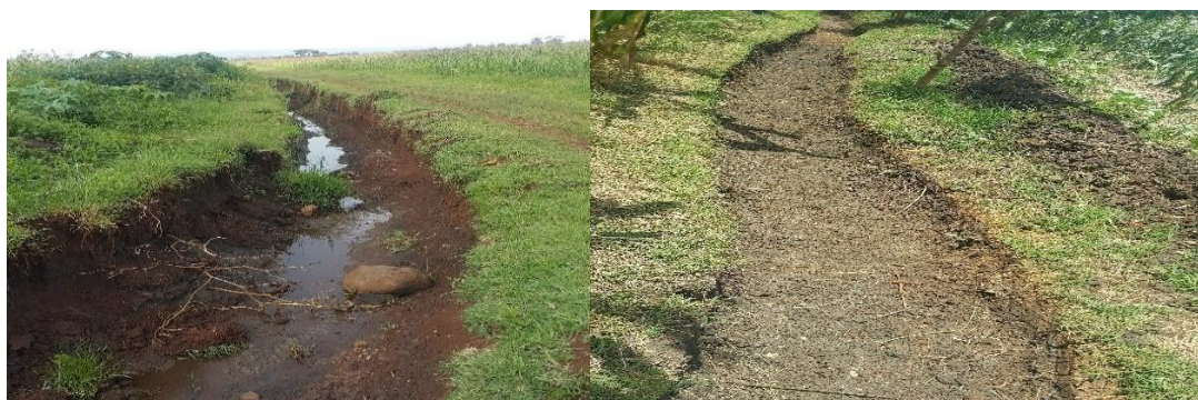
Plate 4.6: Drainage ditches at Amani Scheme during wet season and dry season
