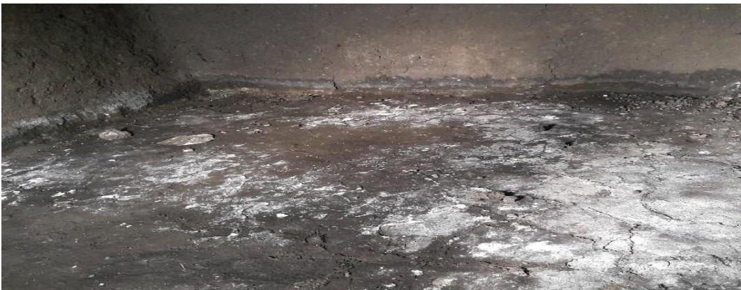
Plate 4.8: Waterlogged house floors due to underground seepage
