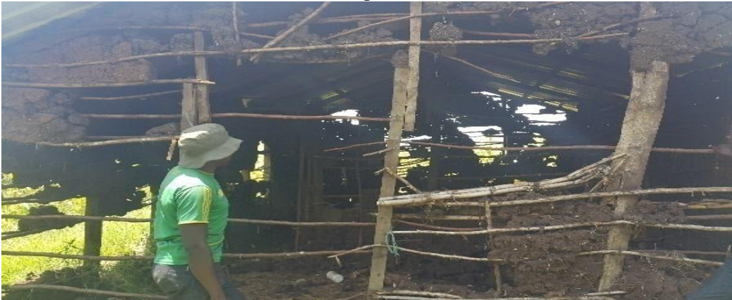
Plate 4.7: Collapsed house walls
