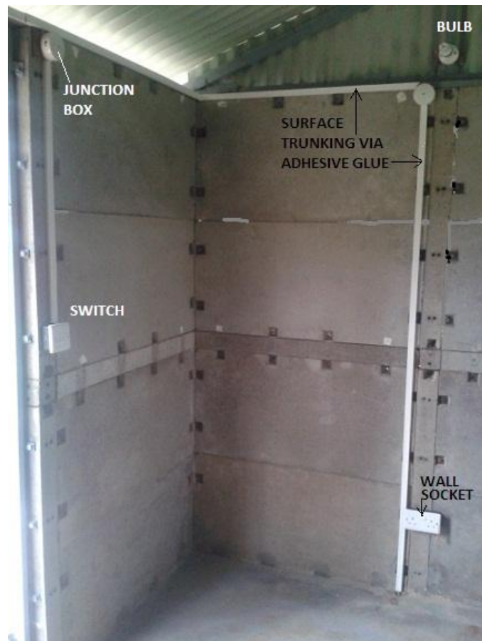
Figure 4.1834: Electrical services incorporated on the surfaces
