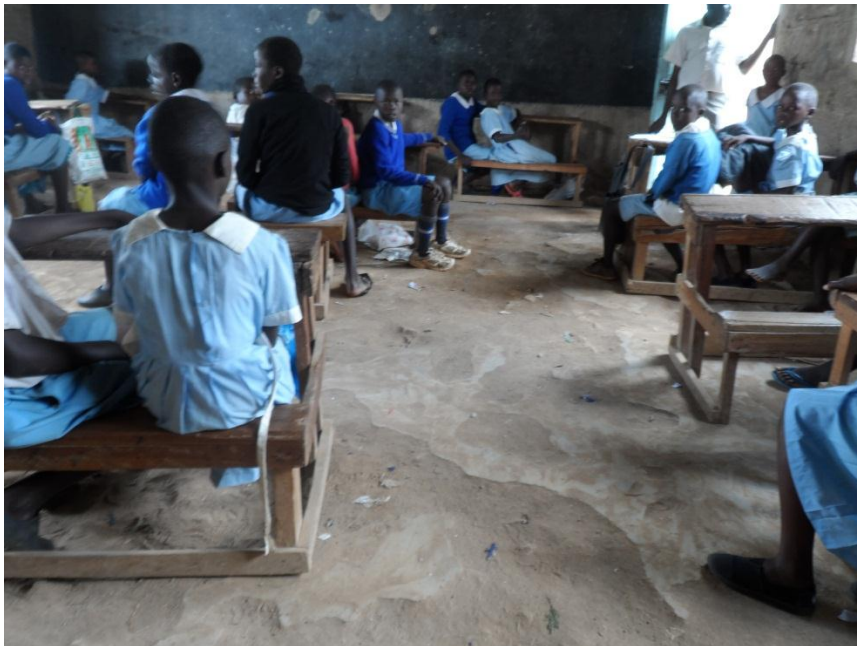
Plate 5: A dilapidated classroom floor in Muyala primary school
