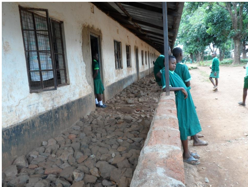
Plate 3: A stalled renovation project in Matende primary school
