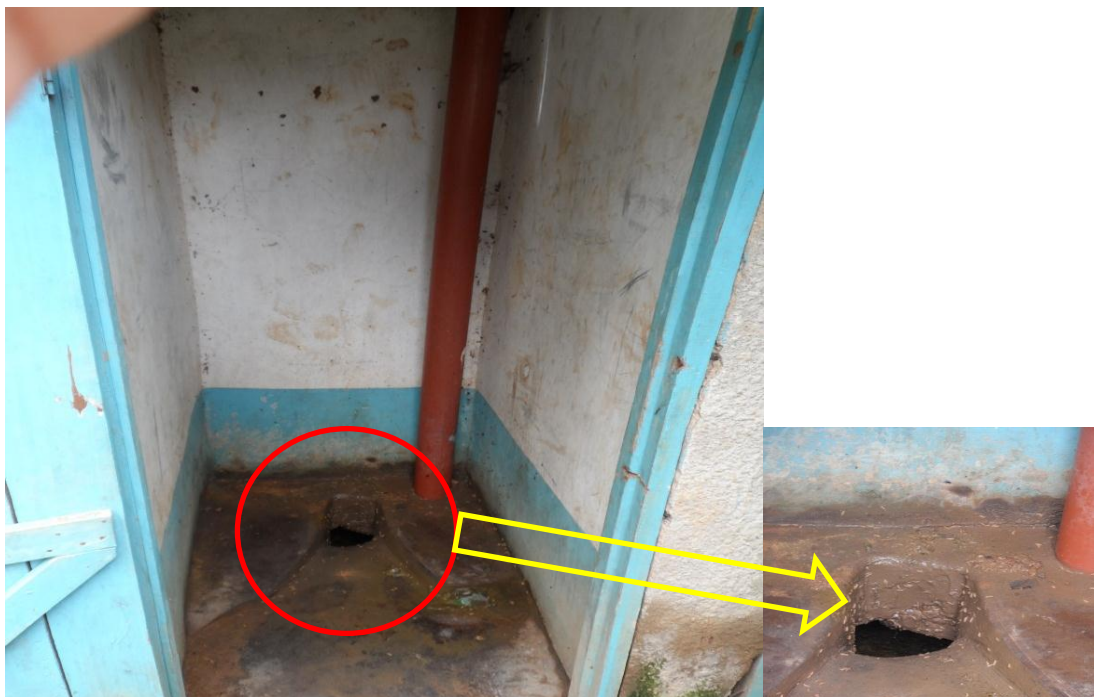
Plate 10: A filled up pit latrine with maggots still in use at Mahiakalo primary school
