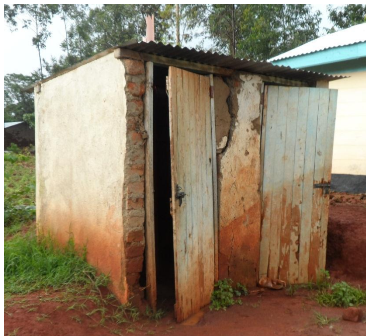
Plate 12: A dilapidated pit latrine in Nyayo Tea Zone primary school
