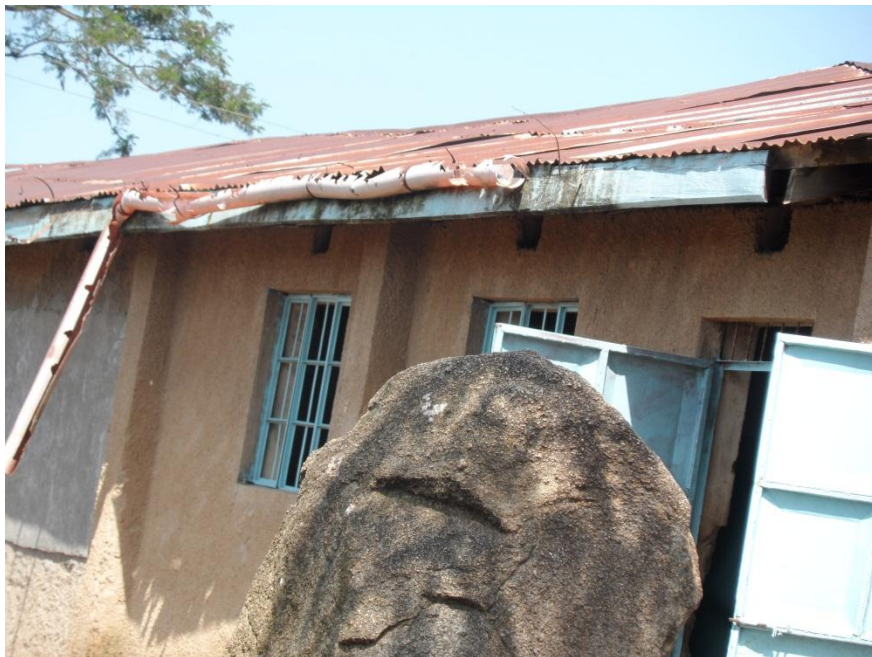
Plate 8: Neglected rain water collection gutters at Ebwambwa primary school
