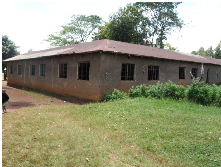
Plate 2: A condemned classroom block that is still in use at Shitaho primary school
