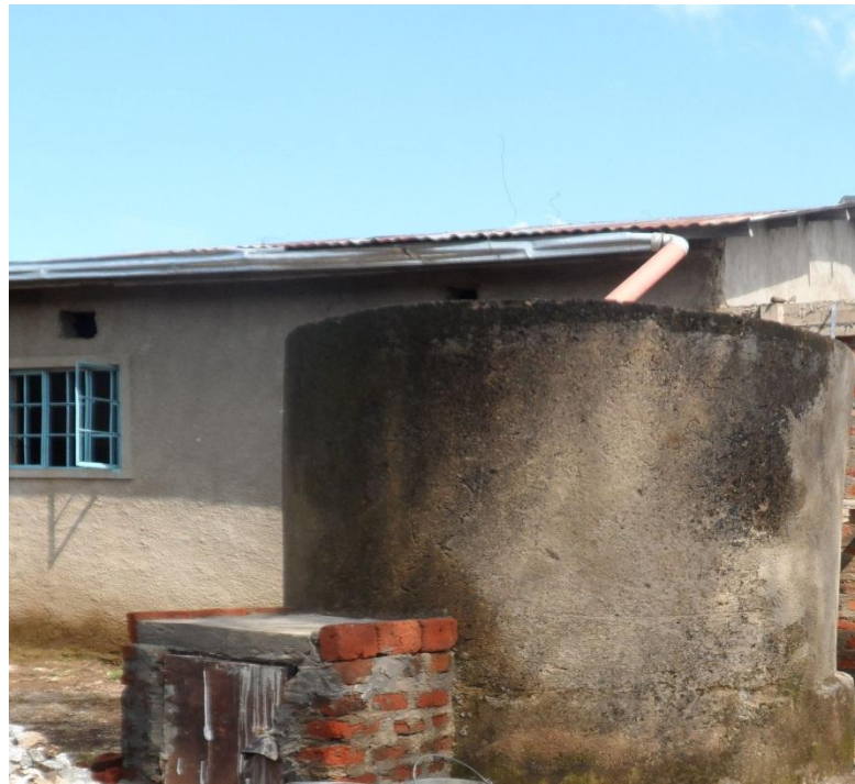
Plate 1: Water conservation tank in Ebwambwa primary school
