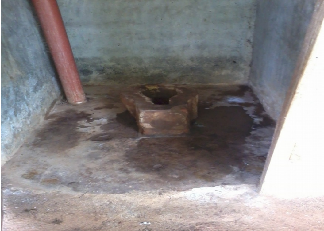
Plate 4.12: A Sullied Adapted Toilet with no Holding Rails
