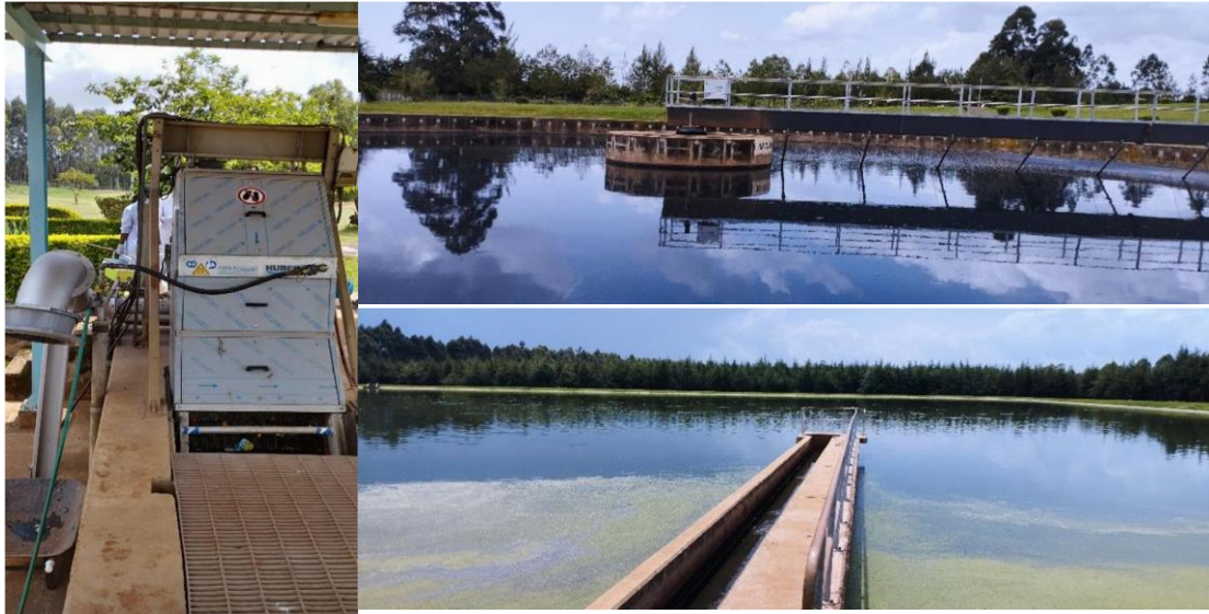
Figure 2: A picture showing the ELDOWAS wastewater treatment plant's physical treatment, trickling filters, and secondary pond.
