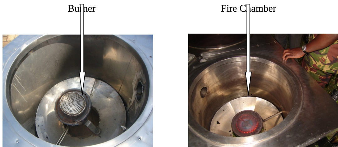
Figure 1.5: Diesel Burner inside the Fire Chamber
