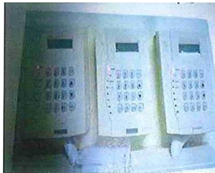
Fig 6: Access control System
