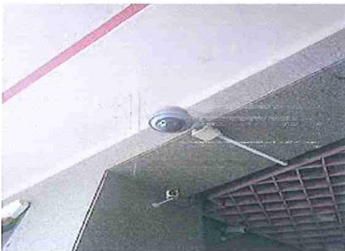
Fig 1 Dome CCTV Camera
