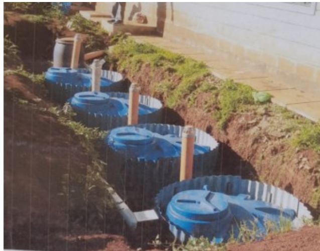
Plate 4.6: System of Bio-San toilet
