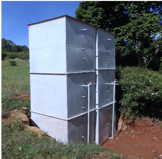
Figure 3.6 Two Slow Sand Filter (SSF) units
