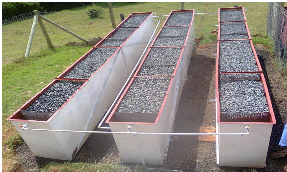
Figure 3.5 Three Horizontal-flow Roughing Filters (HRFs)
