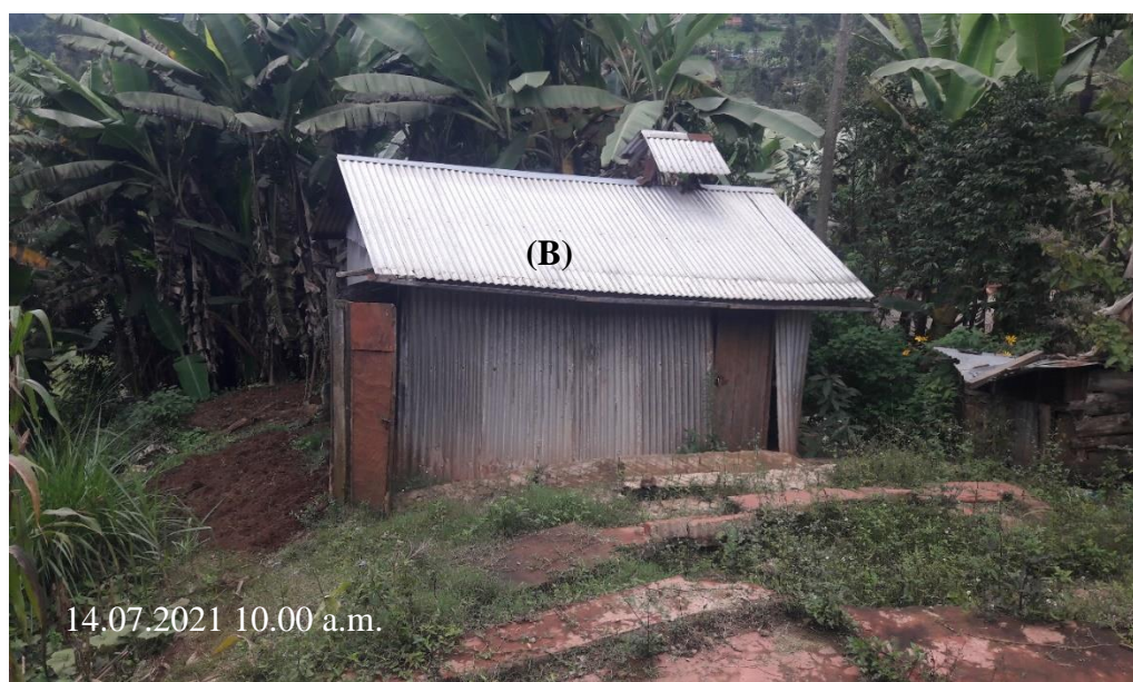
Plate 4.3: Houses abandoned after the year 2018 landslides in Rwathia Location, Kangema Sub-County Source: Field Data
