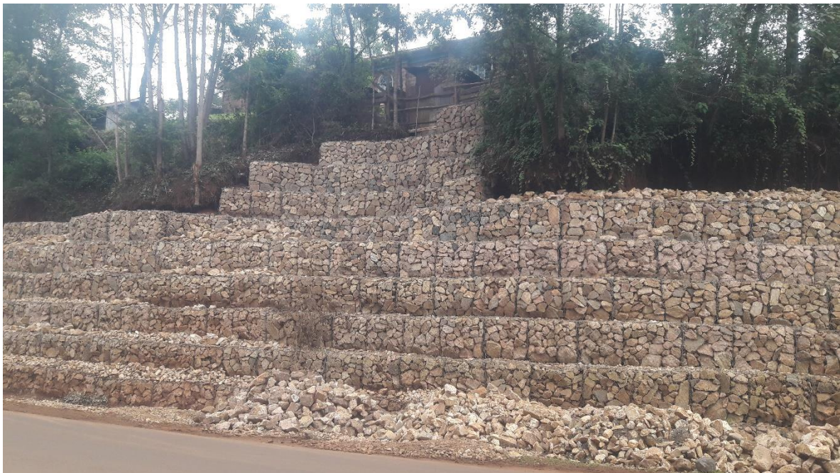
Plate 4.6: Road-side land embankment to prevent further landslides
