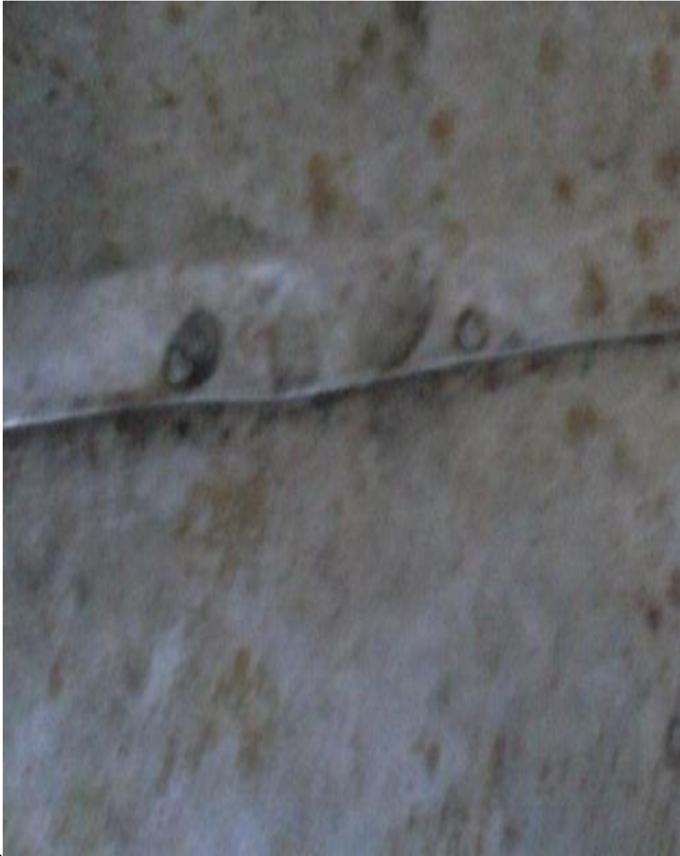
Plate 4.11: Rusted work surface joined with nails
