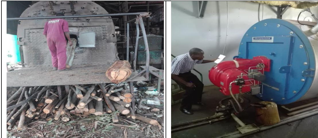
Figure 3.2: (a) Wood fire tube boiler and (b) Thermo boiler used in Rivatex East Africa Ltd
