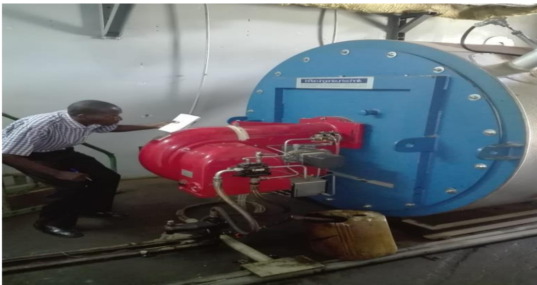
Figure 4.18: Ignition point of Thermo oil boiler
