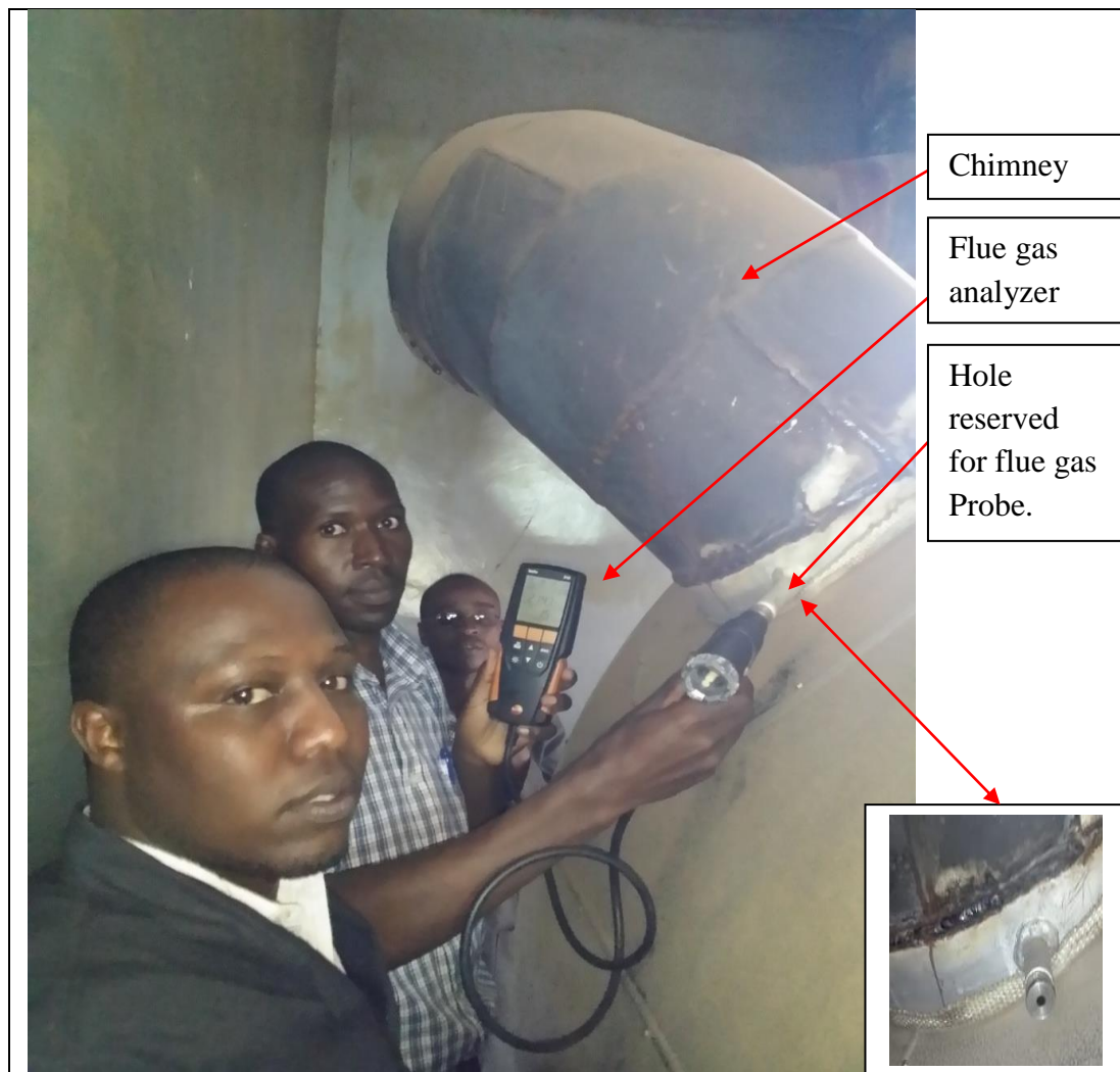
Figure 3.3: Flue gas sampling using flue gas analyzer
