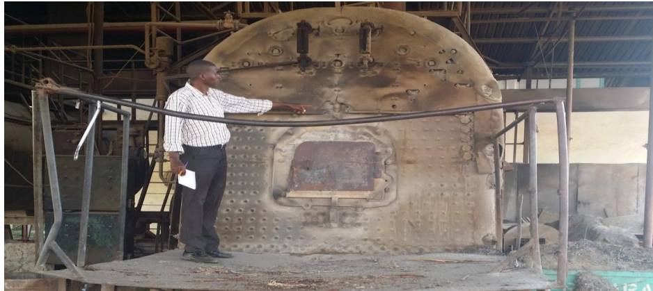
Figure 4.16: Combustion chamber of wood fire-tube boiler
