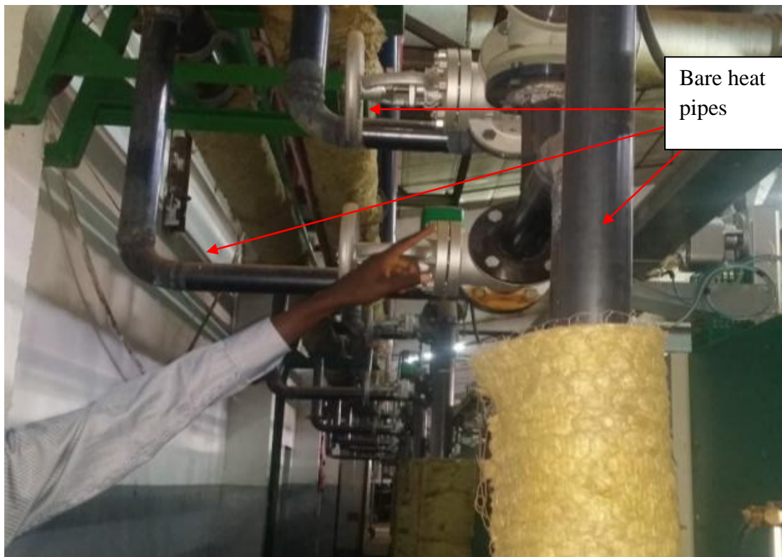
Figure 3.5: Bare (uninsulated) heat distribution systems
