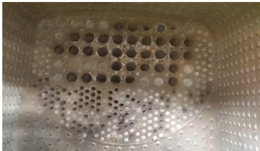
Figure 4.17: Blocked fire tubes of wood fire-tube boiler
