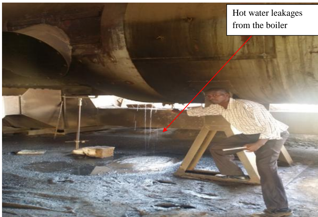
Figure 4.14: Leakages of hot water from wood fire-tube boiler
