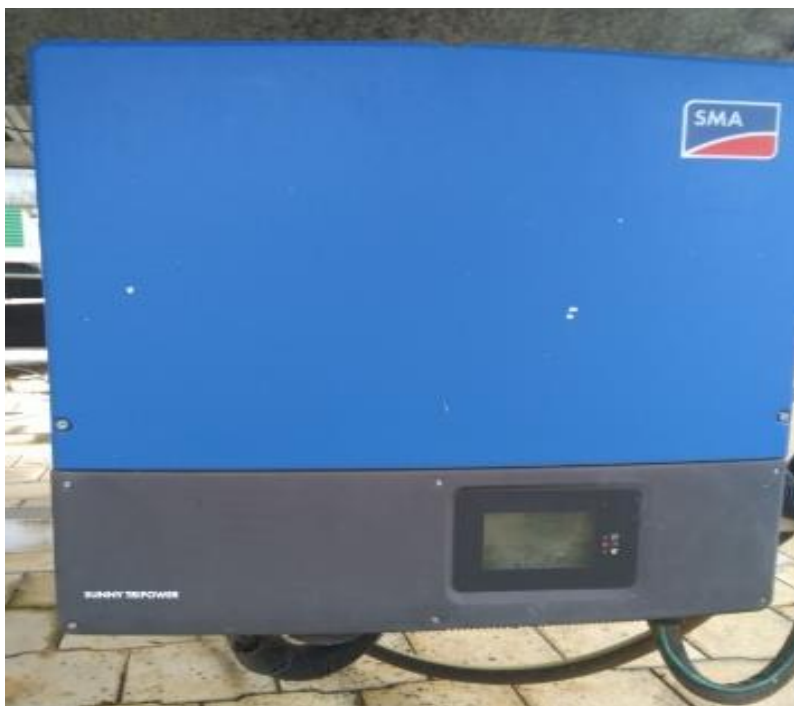
Figure 3.2: SMA Sunny Tri-Power 25000tl Inverter.
