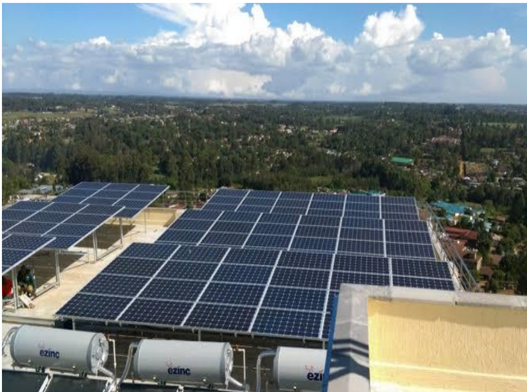
Figure 3.1: Installed Solar Panels on Rooftop of Daima Towers
