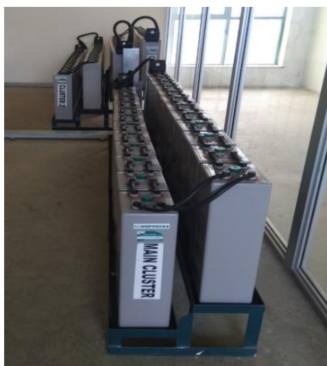
Figure 3.4: Valve Regulated Lead-Acid OPzV Batteries.
