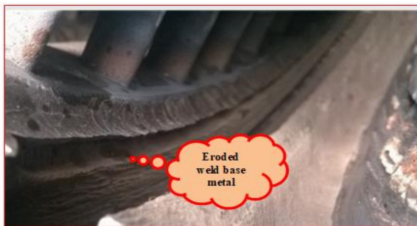
Figure 1.2: Eroded diaphragm base (Source: Researcher, 2019)
