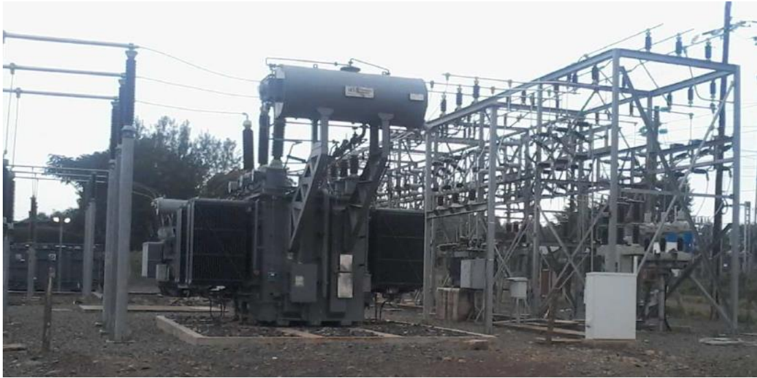
Figure 1.1: Lessos 232/33 KV, Substation 23MVA TX (KPLC, 2020.)
