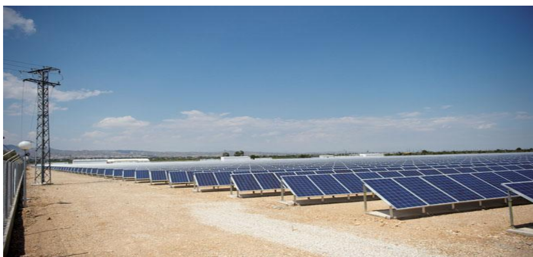
Figure 2.4: Ground mounted grid tie PV (Source: SMA Solar Technology AG, 2017)
