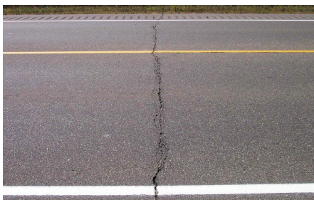
(a) Transverse cracking
