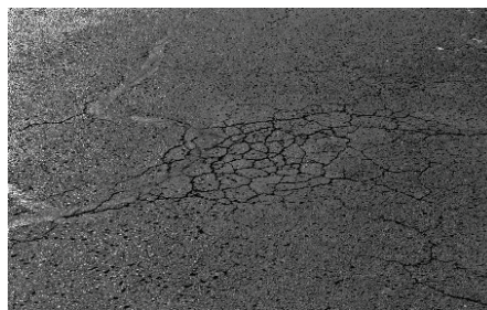
(b) Alligator (fatigue) cracking
