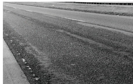
(e) Raveling-microtextural surface deformations
