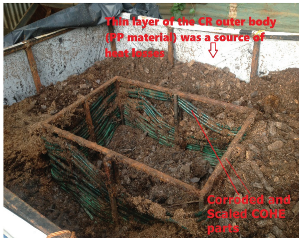
Figure 12. Scaled up and corroded COHE parts.
